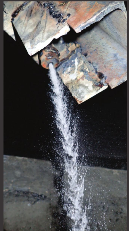
Picture 3 and 4: Wrong nozzle and dust collection
